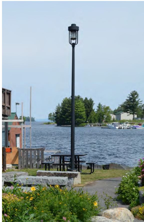
Existing pedestrian light fixture in Thoreau Park
